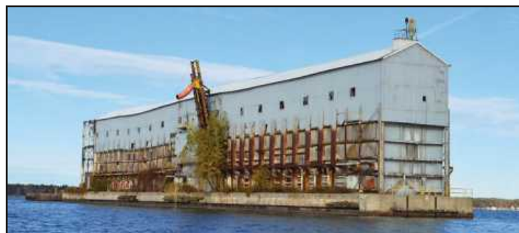
LONG ABANDONED, the Alabaster marine bin which distributed gypsum to ships was demolished in 2020. The conveyor system which fed it “represented a compromise between a major dredging operation to allow freighters to transport gypsum out of Alabaster and barging the material to freighters in deep water,” says the website Abandoned . “The ships took gypsum from Alabaster to East Chicago, Indiana or Detroit for manufacture into various gypsum products.” Photo credit: USG
