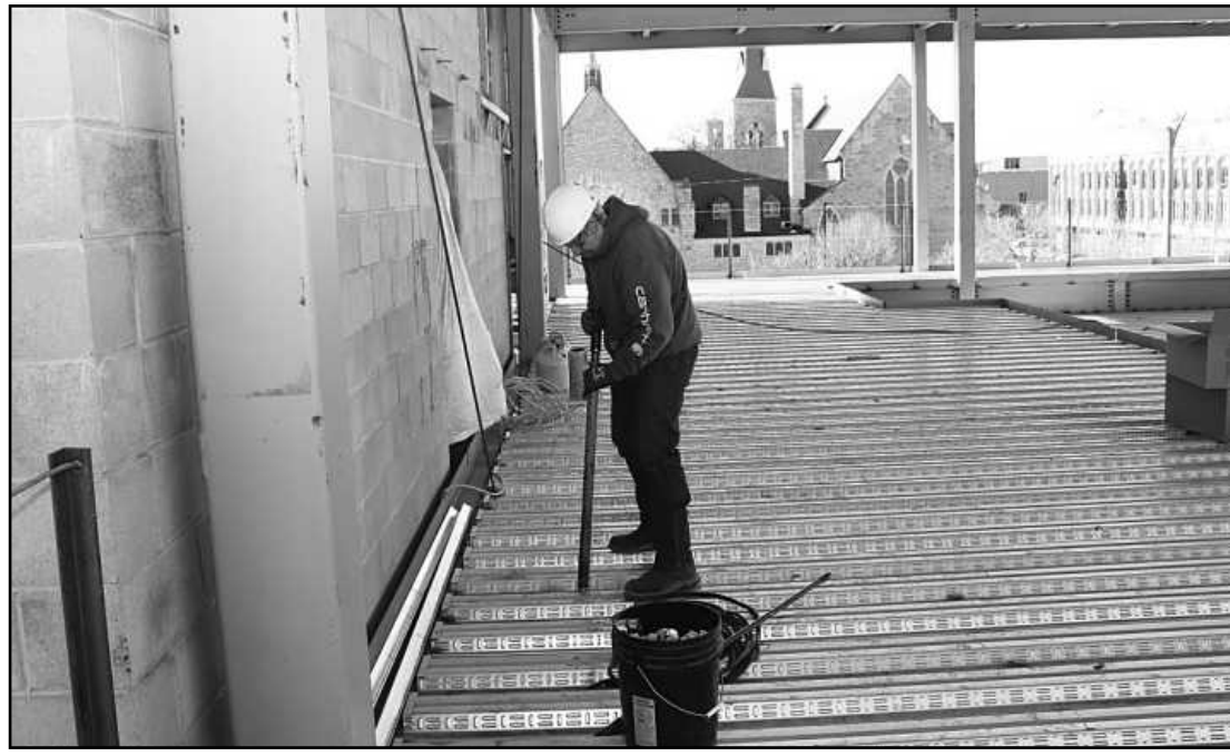
PUNCHING HOLES to allow for the setting of duct hangers below is Ken Krupp of Sheet Metal Workers Local 7. He’s employed by Dee Cramer, working at the Harrison Street Commons project in Flint.
