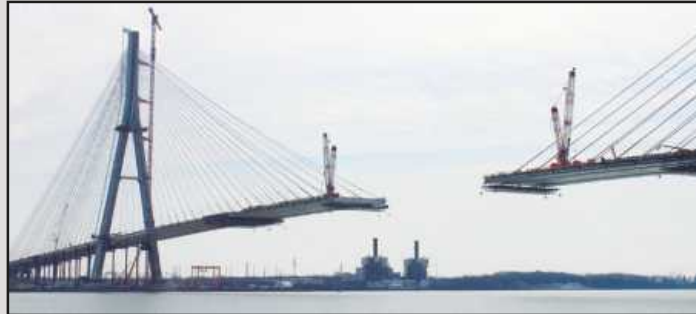
THE CURRENT GAP in the Gordie Howe Bridge is less than 500 feet, and Windsor and Detroit tradespeople are expected to be shaking hands when the deck sections are connected by the end of this summer. The main span is 138 feet above the Detroit River near the towers, and with a 5 percent incline, it will reach 150 feet in the middle of the river.
