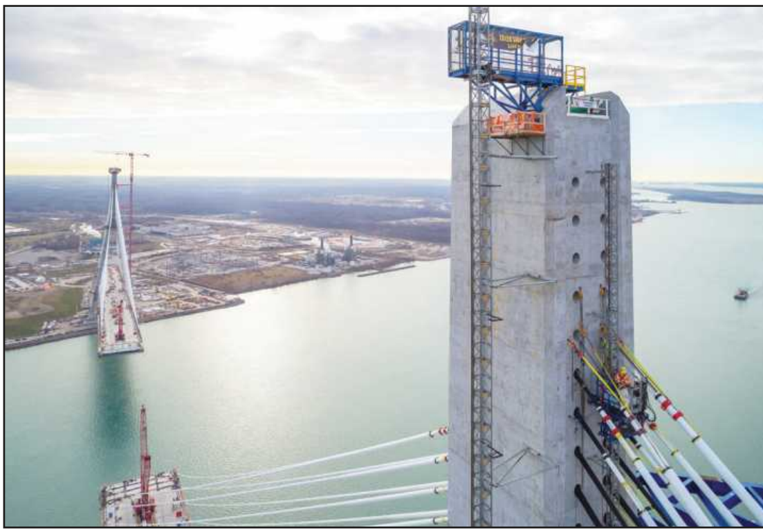
STAY CABLES on the Detroit side of the Gordie Howe Bridge support the full weight of the bridge deck. The cables are comprised of rope-like metal strands housed in a high-density polyethylene plastic pipe. A total of 3,107 miles of stay cables are being used to support the span.
