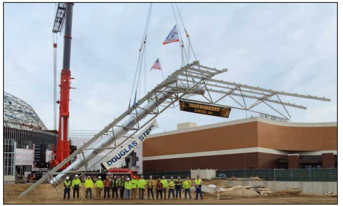
IRON WORKERS Local 25 members employed by Douglas Steel gather under the final section of steel ready for placement at the Aquadome at the Gun Lake Casino hotel. Photo credit: Ben Roberts
