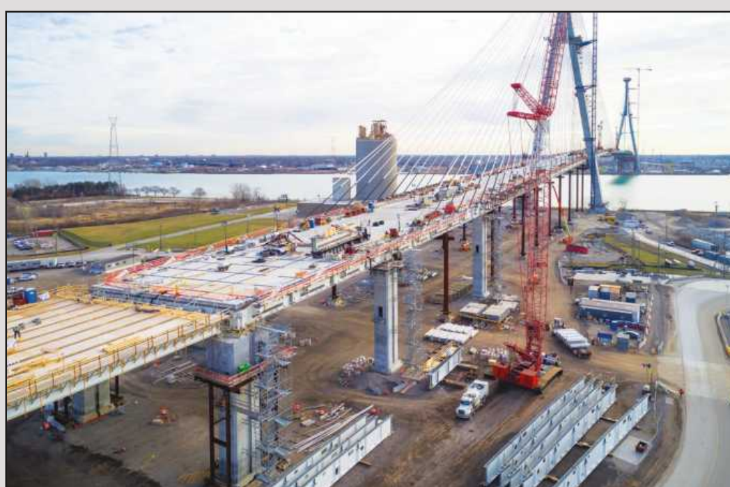
BUILDING TRADES WORKERS are making rapid progress on erecting the Gordie Howe Bridge connecting Detroit and Windsor, Ontario. The 722-foot-tall towers and the six-lane bridge deck over the Detroit River are the most visible portions of the project, but there is also a tremendous amount of work "back bridge" in Southwest Detroit, with Point of Entry structures, overpass and other road work.
