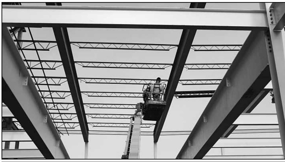
ERECTING STEEL in what will be the YMCA portion of the Harrison Street Commons project in Flint is Chad Oliver of Iron Workers Local 25. He's employed by AMS Steel.
