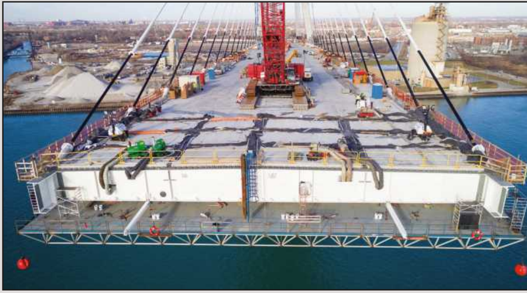
THE GORDIE HOWE BRIDGE'S leading edge of its main span is shown, looking at Detroit. The span is constructed one segment at a time, with the cables tied to the tower and main span tied back to the already completed approach span. Deck construction follows shortly behind the steel, and a crawler crane services both tasks from the deck. The superstructure is built of structural steel edge girders and floor beams with a composite, precast panel deck.
